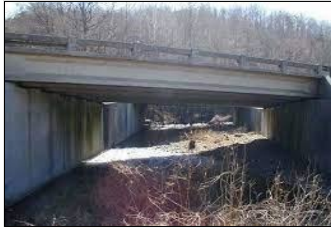
Figure 2-13. Bridge underpass along I-81 north of Buchanan used as a wildlife crossing. (VTRC 2022)
